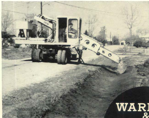
Gradall® , a machine of many jobs, digging drainage ditches in a southern town.
