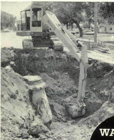
The Hopto® 500 hydraulic backhoe working on a sewer project in a midwestern town.
