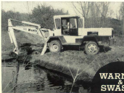
The Hopto® hydraulic backhoe digging a drainage trench for a southern construction company.
