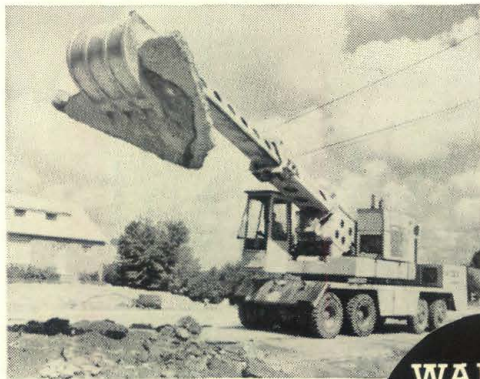
The big G-1000 Gradall® ripping concrete on a new midwestern highway project.
